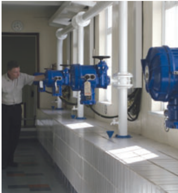
Filter controls at Handois Treatment Works
