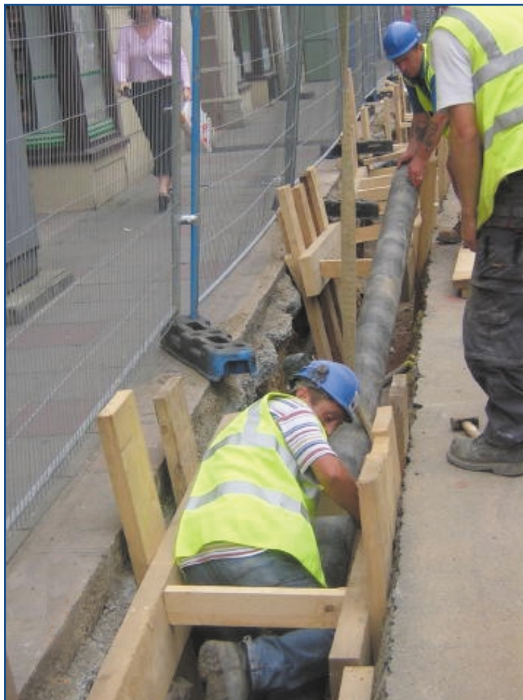
John Le Guilcher, Foreman Mainlayer (in the foreground) and his team laying a replacement 150mm diameter water main in Union Street, St Helier
