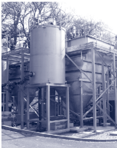
Handois Wash Water Recovery Plant
