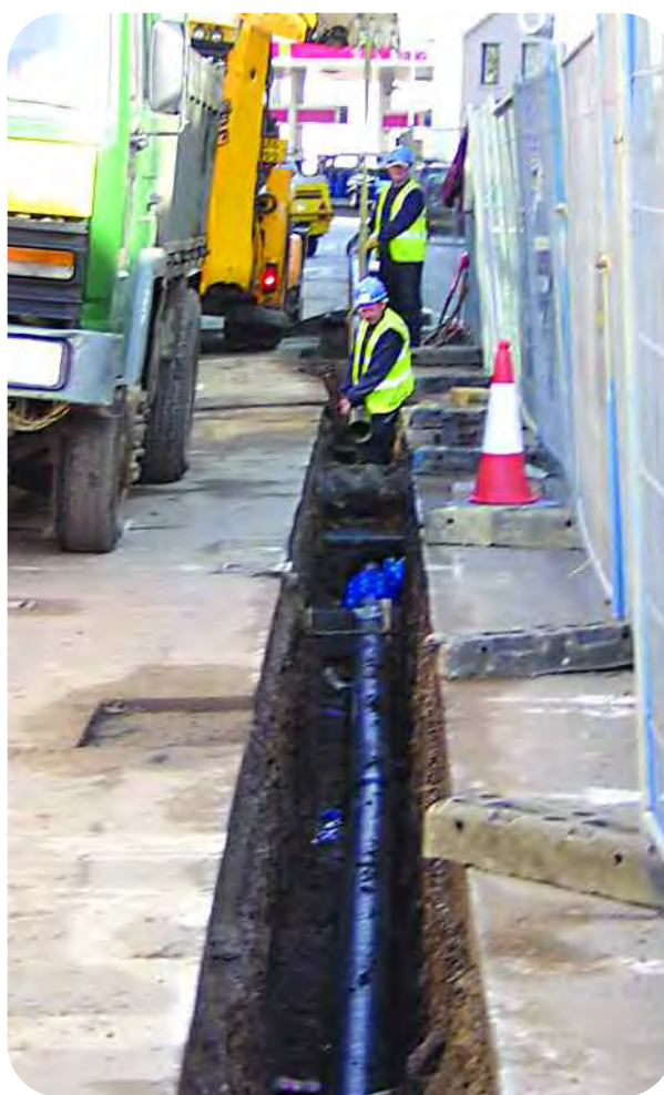
Foreman Kevin Bassett and Joe McGowan laying a replacement 150mm diameter water main in St Helier
