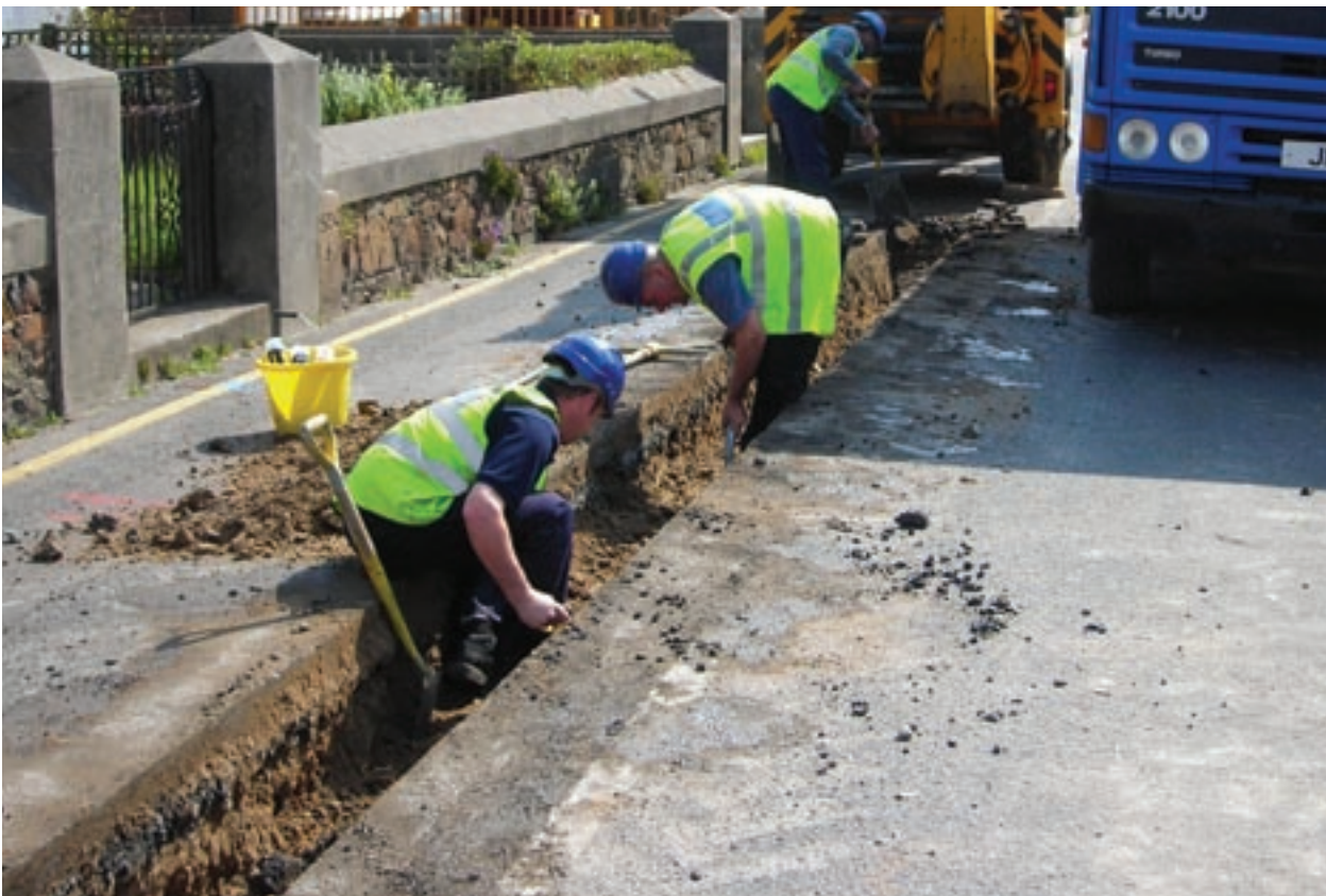
During the year some 5.5 km of new water mains were laid and 1.98 km of water mains were replaced.
