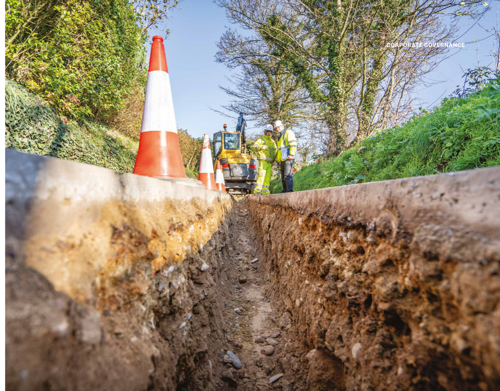
Craig Balyckij, Water Network Controller and Iain Samson, Network Supervisor
